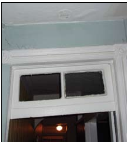
Figure 1: Cracks over doors or floor/frame misalignments are usually good indicators of settlement problems.
