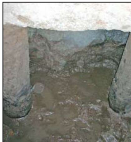
Figure 2: To access the piles, dewatering is often required. Depending on the pit size, only a limited number of piles can be accessed.
