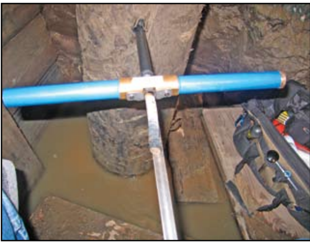
Figure 4: Due to limited access to piles, only a limited number of cores can be obtained.
