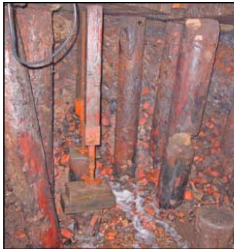
Figure 5: Removal is often difficult because the pile may be carrying significant load. The underside of the pile cap may require shoring to maintain stability.
