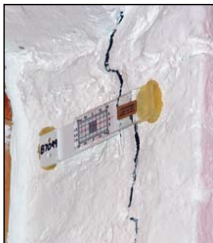
Figure 1: Crack gauge is placed across an existing crack to monitor future movement.
