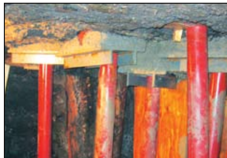
Figure 4: Steel pipes are inserted to fully replace the deteriorated portion of the pile. The void is later filled with concrete.
