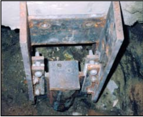
Figure 6: Push-pier pile is installed with a steel bracket tucked in under the foundation pile cap.
