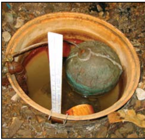
Figure 3: An automated device controlling groundwater table – the recharge system “kicks in” when water elevation drops below a predetermined level.
